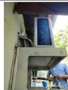
12-HT - Quarto 01 Agratto 18K N/A equipamento instalado 09° 38' 7.6" S 35° 44' 6.0" W - 10/09/2025 15:47
