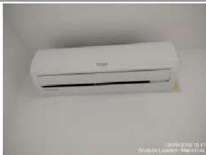
11-HT - Quarto 01 Agratto 18K N/A equipamento instalado 09° 38' 8.2" S 35° 44' 8.0" W - 10/09/2025 15:47
